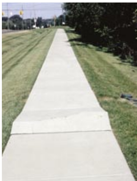
This hot summer day, cracking the sidewalk
