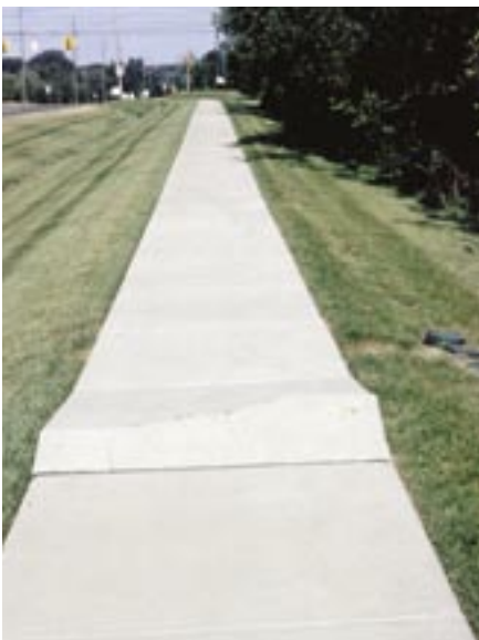
This hot summer day, cracking the sidewalk
